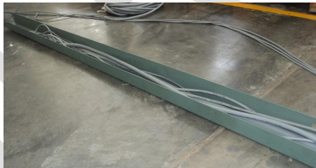
Fig 1: Cables carrying Cable Duct
