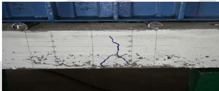
Fig.20 Crack pattern for 100G5 of M40
